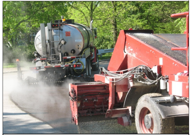
Crews apply a new coat of asphalt sealer to St. Paul Drive
